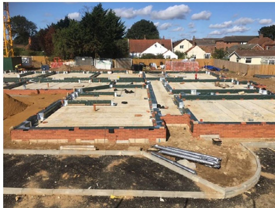
Figure C5 Perimeter cavity membrane with main infill membrane - perimeter cavity gas resistant membrane / DPC
