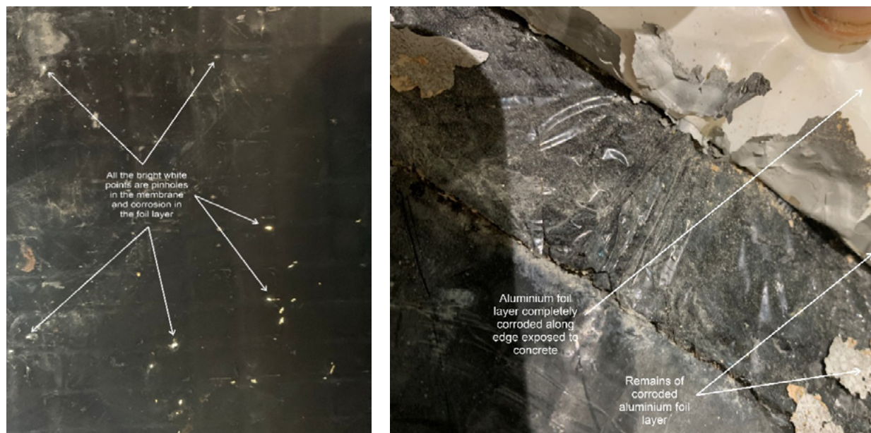
Figure 5.2 (left) corroded foil in a self adhesive membrane (right) corrosion pin pricks in a membrane
